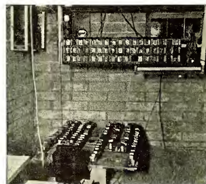
Fig. 2—The Plate Supply, in the Basement
