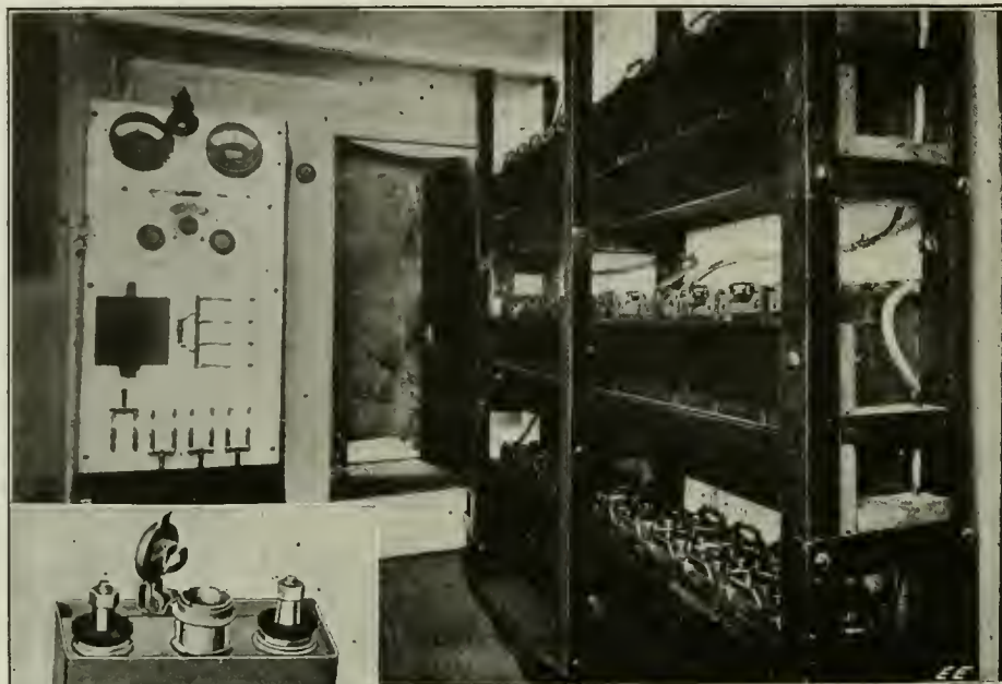
A Typical Alkaline Storage Battery Installation On Ship-Board, the Battery Operating the Wireless Telegraph Equipment In Emergency. The Control and Charging Switch-Board Appear At the Left of the "Battery Room." All Radio Operators Should Thoroughly Understand Storage Batteries, Both the Lead and Alkaline Types. The Smaller Cut Shows the Non-Leaking Gas Vent Fitted On the Alkaline Cell. This Cell Has a Mean Potential of 1.2 Volts.
