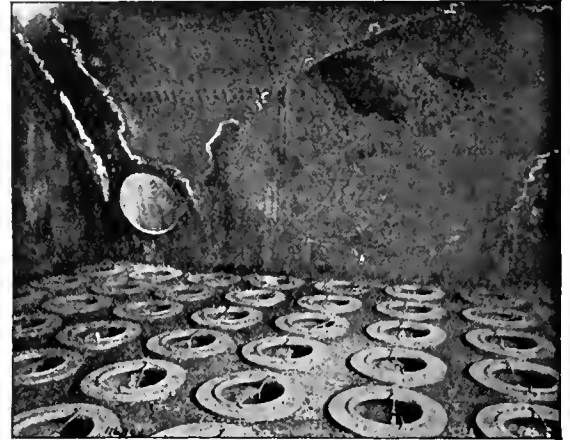
Interior of High Tension, Direct Current, Electrode Chamber Inside of Flue Tube Measuring 13 Feet in Diameter. The Electrodes Are Suspended Chains Which Carry the Charge When in Use.
