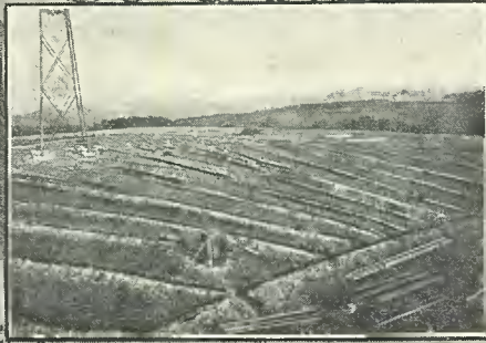
The excavations for the construction of the elaborate ground system, showing the trenches for the heavy ground wires. They cover radially a huge ellipse.
