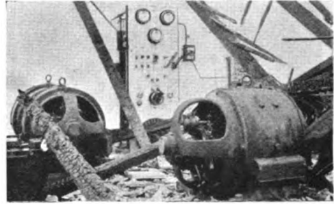
The Wrecked Generators at Duala.
